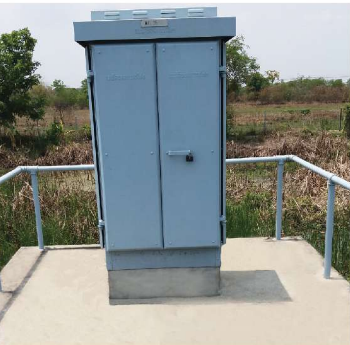
“Signal and Location Cabinet”
