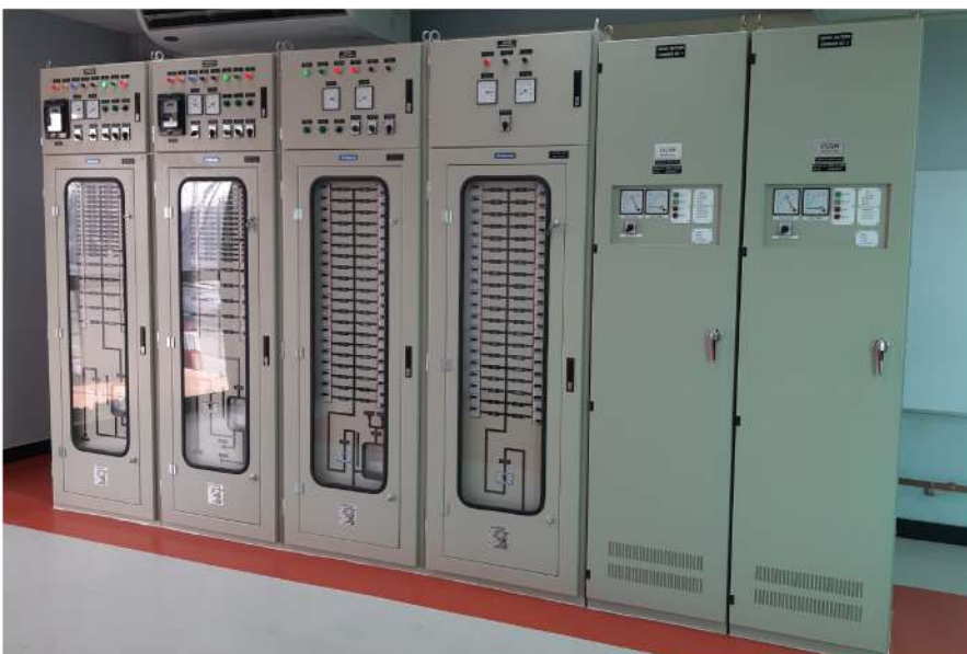
“AC-DC DISTRIBUTION BOARD AND 125 VDC BATTERY CHARGER” 22 kV SUBSTATION
