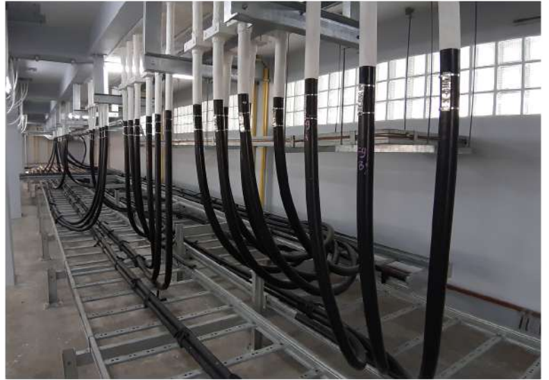
“H.V. POWER CABLE 22 kV SUBSTATION”
