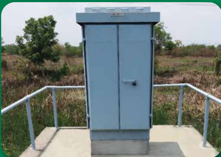
SIGNAL CONTROL CABINET
